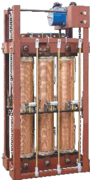
Regulator View of Rectifier
